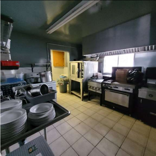
Figure 7-10: Industrial Kitchen with Hood Vents
