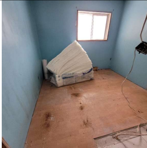
Figure 7-8: Incomplete renovations. Loose Electrical
