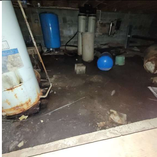
Figure 7-9: Water tanks in basement
